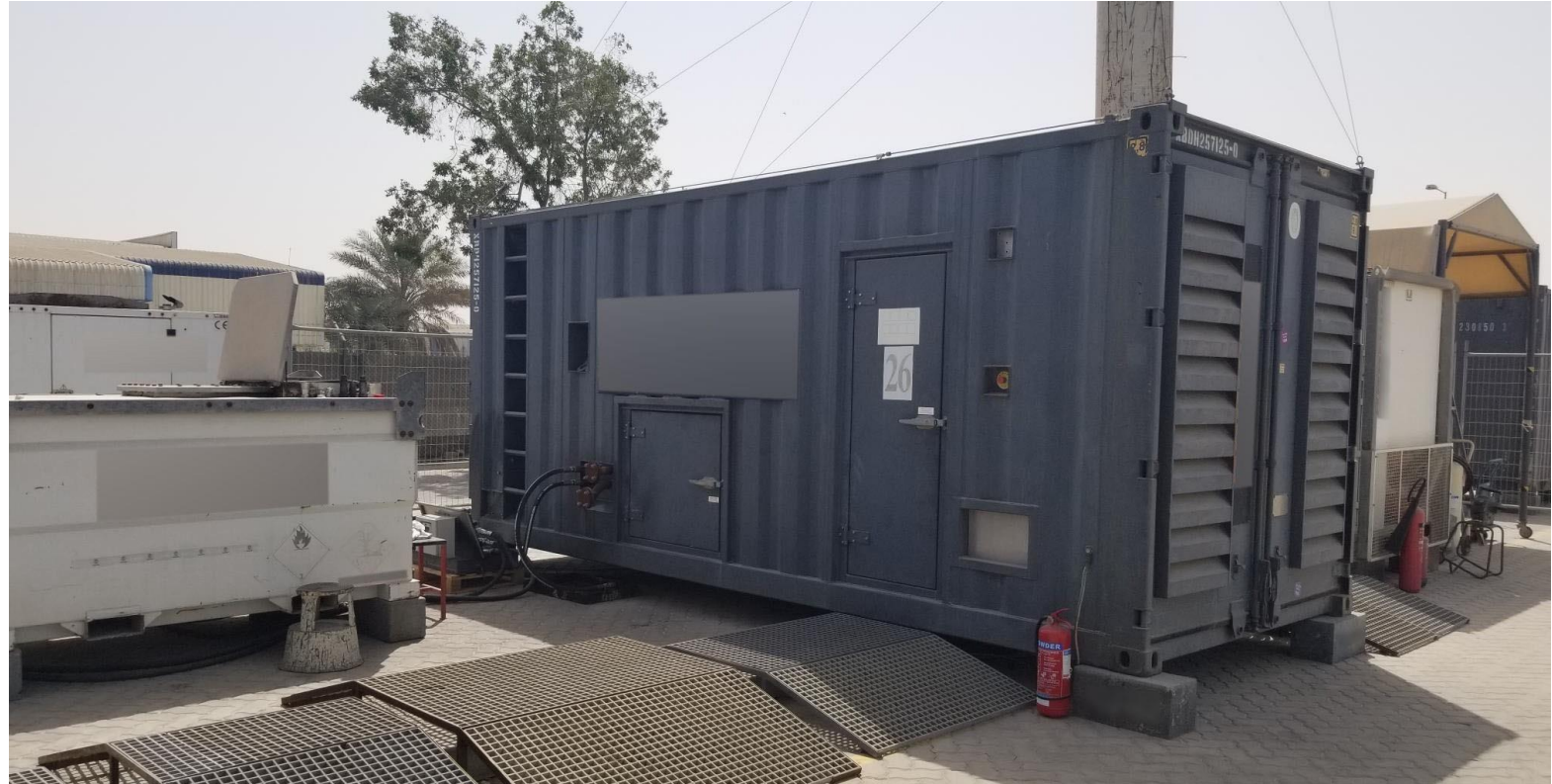
Fuel Tank and Containerised Generator
